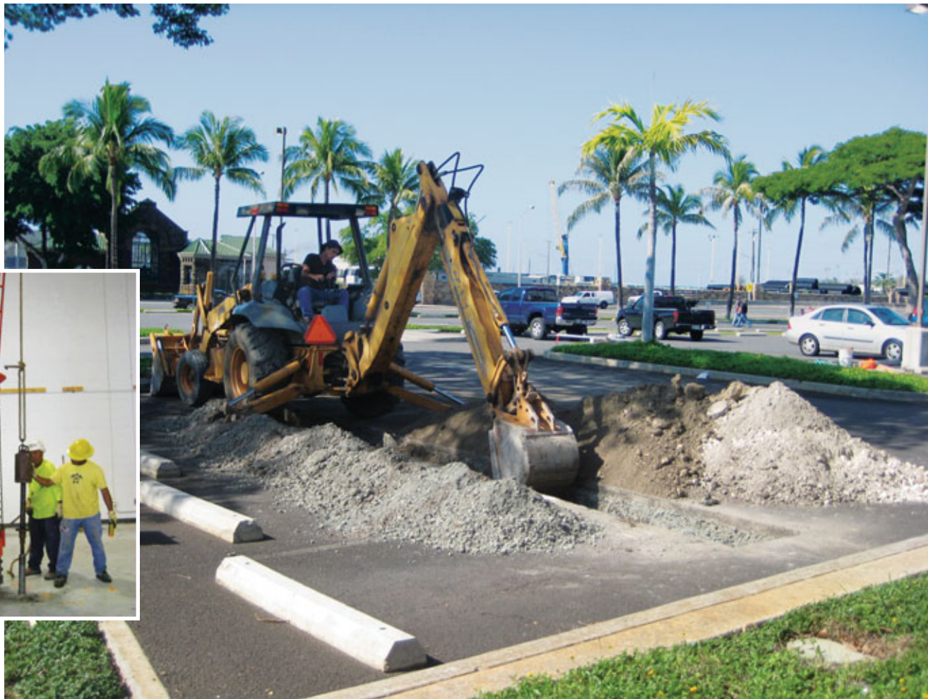
Mike Masutani of Mike’s Backhoe excavates a trench for the Archaeological Inventory Survey at the former CompUSA site in Kaka’ako. Inset: core samples are taken from inside the former CompUSA building.
